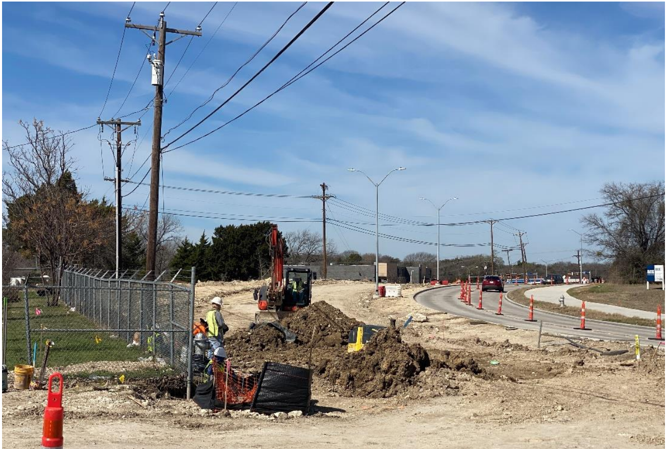
Danieldale Rd. - Verifying utility depths
